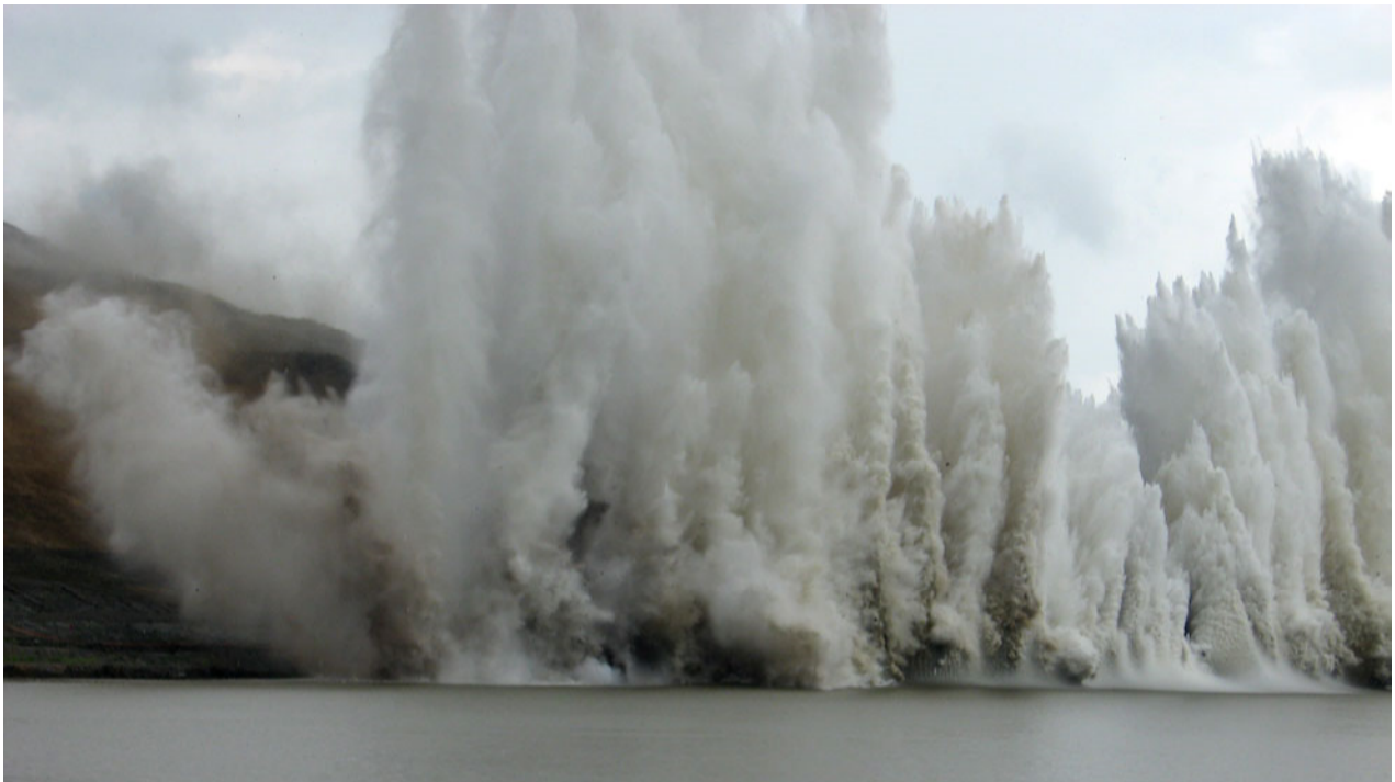
The first explosions marking the beginning of the expansion project for the Panama Canal.
