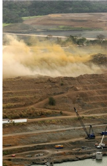
Controlled explosions in Paraiso Hills that are part of the Panama Canal expansion.
